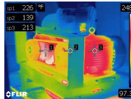
Thermal Image of Overheated Blower Motor at Valentine WWTF
